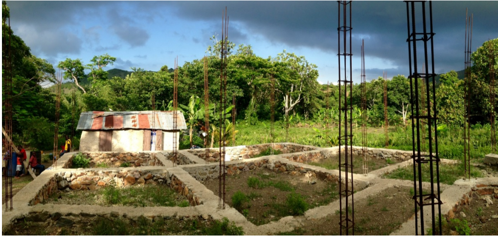
In the foreground is the foundation for the new home of a worker allowed to work in the US in 2015, under construction in 2016 for his family of seven. In the background, his current two-room home. Taken May 22, 2016 in Milot, Nord by Hannah Postel.
