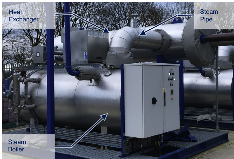
Fig. 4. Site photo of the immersion tube thermosyphon heater (ITTH).
