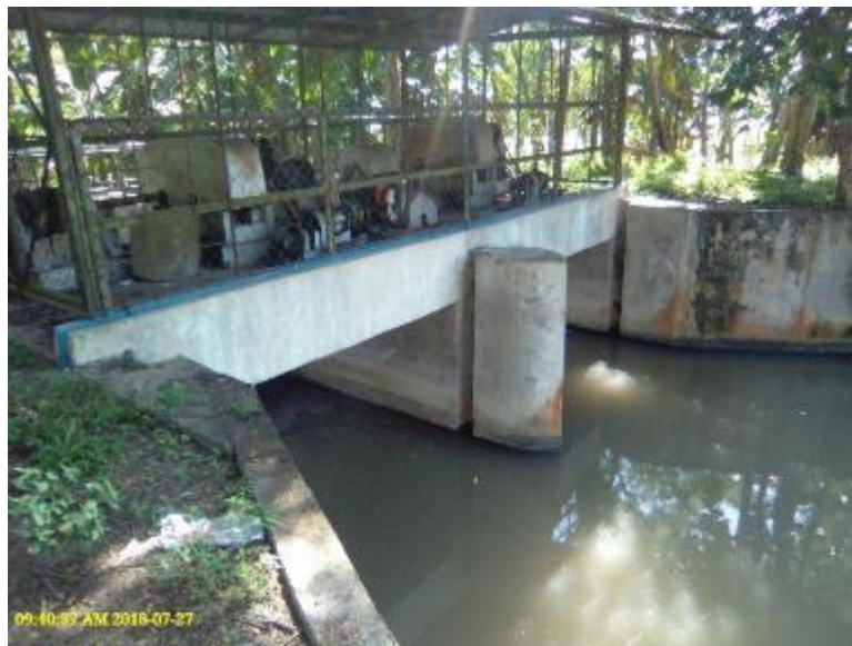
Photo 87. Control gates of the silt ejector of Marbel #1 RIS.
