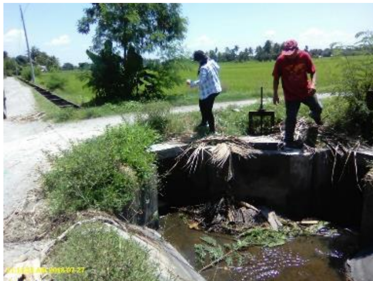
Photo 85. Section of Main Canal of Marbel #1 RIS at the headgate of Lateral H1.
