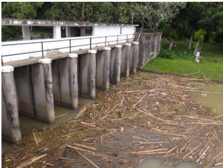
Photo 45. Dry log debris on the side of Jalaur-Suage RIS
