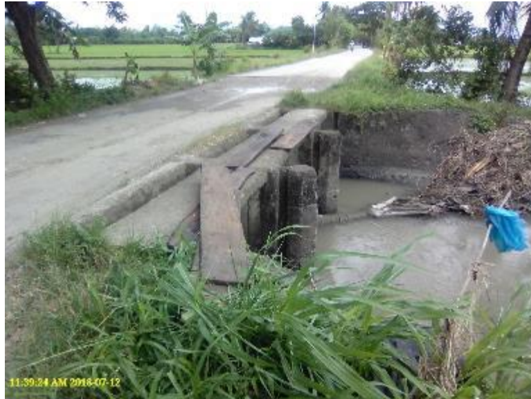
Photo 63. A checkgate using wood planks near the downstream of Main Canal of Jalaur Proper RIS. Take note of the debris on the right side of the canal.
