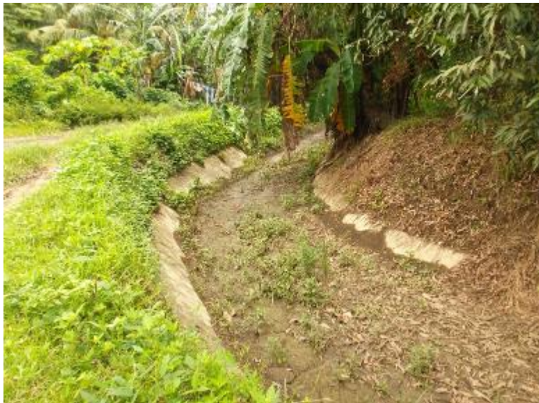
Photo 48. Silted section of Lateral C, Jalaur Proper RIS near the headgate.
