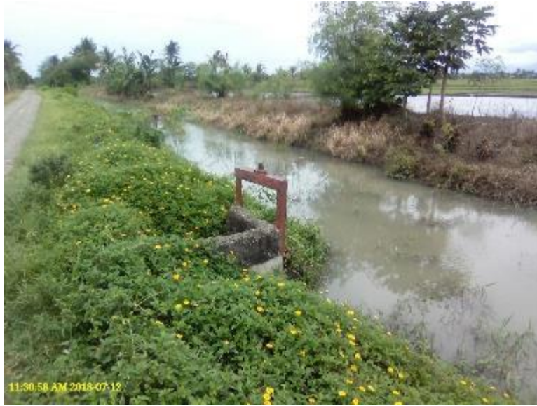
Photo 61. A direct turnout in the midstream of Main Canal of Jalaur Proper RIS.
