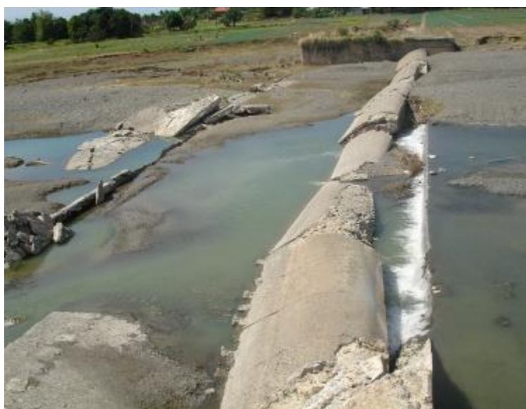
Photo 24. LTRIS dam damaged due to Typhoon Mario
