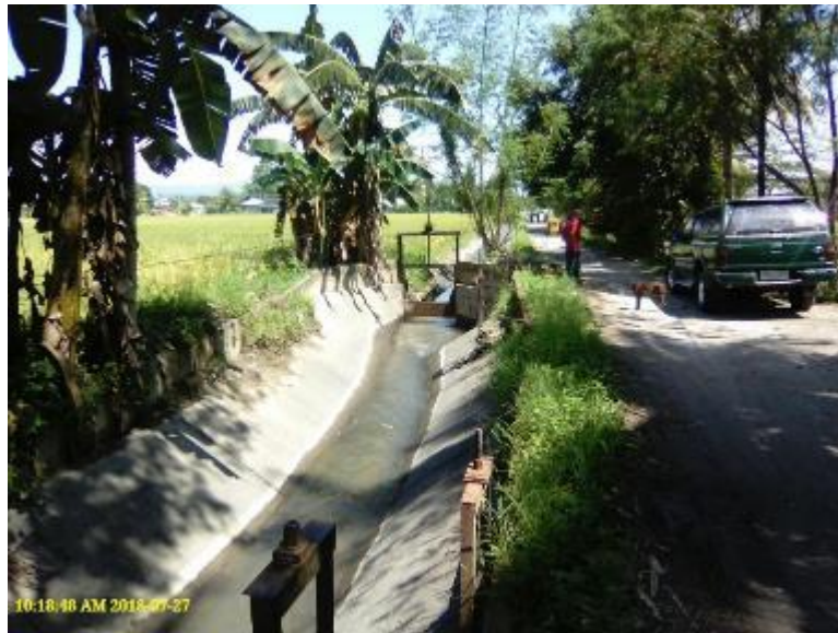
Photo 84. Section of Main Canal of Marbel #1 RIS at the headgate of Lateral E.
