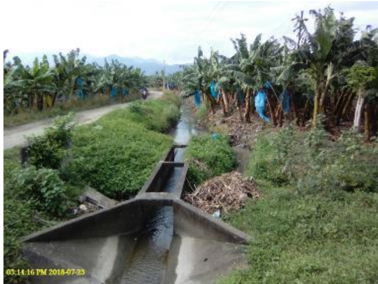
Photo 76. Portion of lined section followed by unlined section in the downstream of Padada RIS.
