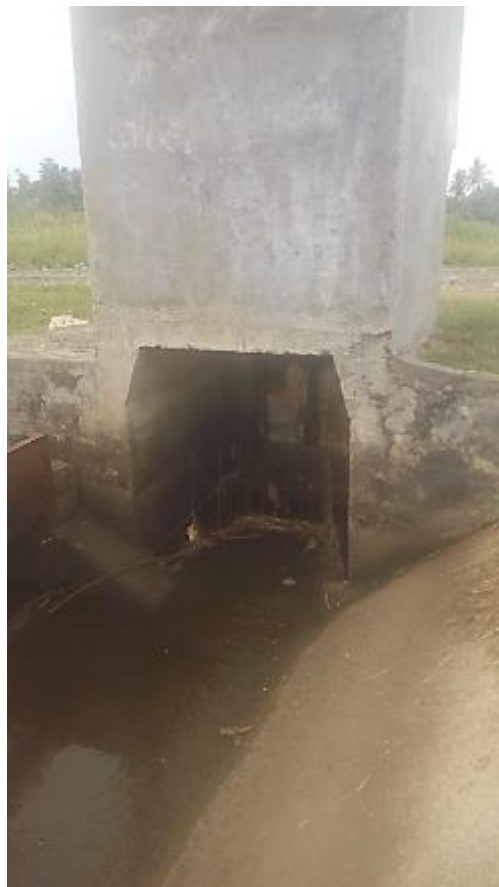
Photo 41. Damaged structure in Malinao IS.
