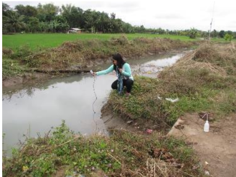
Photo 3. Damaged canal end section of Lateral D2-D2, Div. 4, MARIIS. Pile of sediments could be observed in both embankments of the canal
