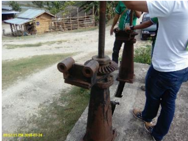
Photo 5. Missing gates in MalMar 2 RIS.
