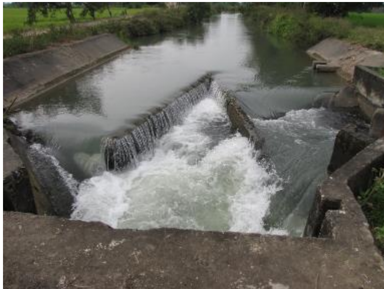
Photo 30. Control and division structures along Lateral B, Div.2, MARIIS. Take note of the damages and condition of the canal and structures.
