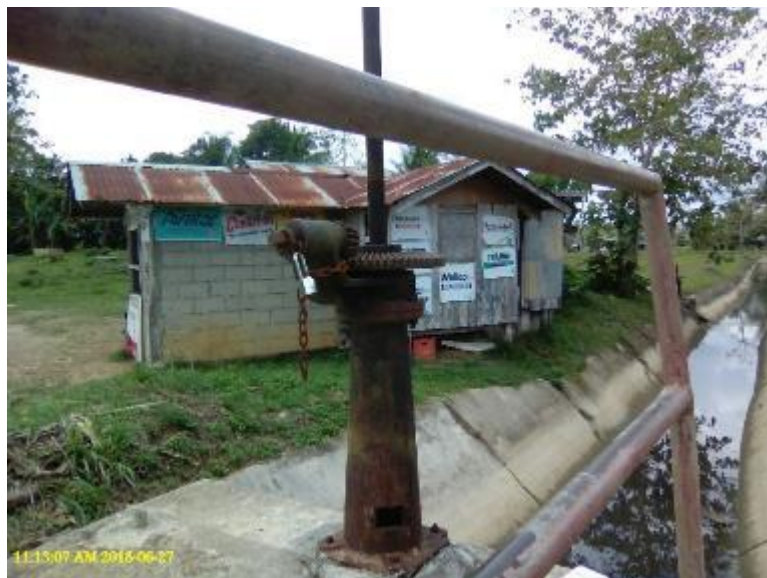
Photo 39. A gate with padlock in the downstream section of Malinao IS Lateral F.
