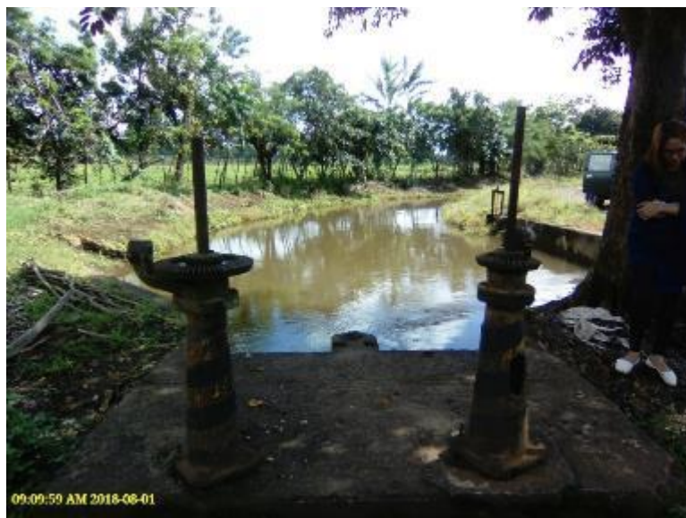
Photo 6. Damaged headgates control lever of Lateral A of Manupali RIS.
