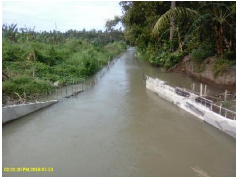
Photo 93. Unfinished construction of Main canal of Padada RIS.
