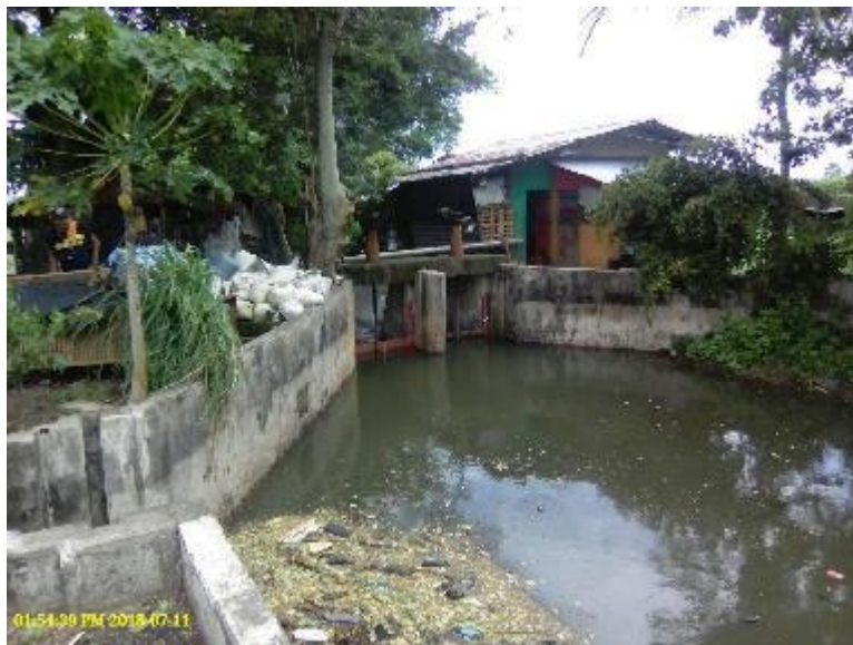
Photo 52. Checkgates at Lateral F, Jalaar Extension RIS. Take note of the floating debris on the left side.
