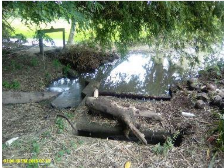
Photo 65. A re-use dam in Suague RIS. The intake gate is on the left side covered with debris.
