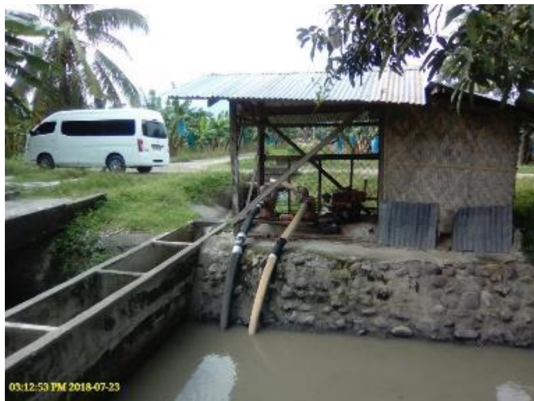
Photo 77. Pump house beside a reuse point in Padada RIS.
