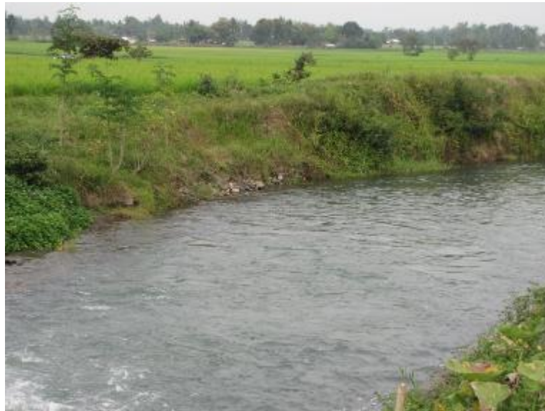
Photo 26. Unlined section of Lateral B, Div. 2, MARIIS with damages from erosion
