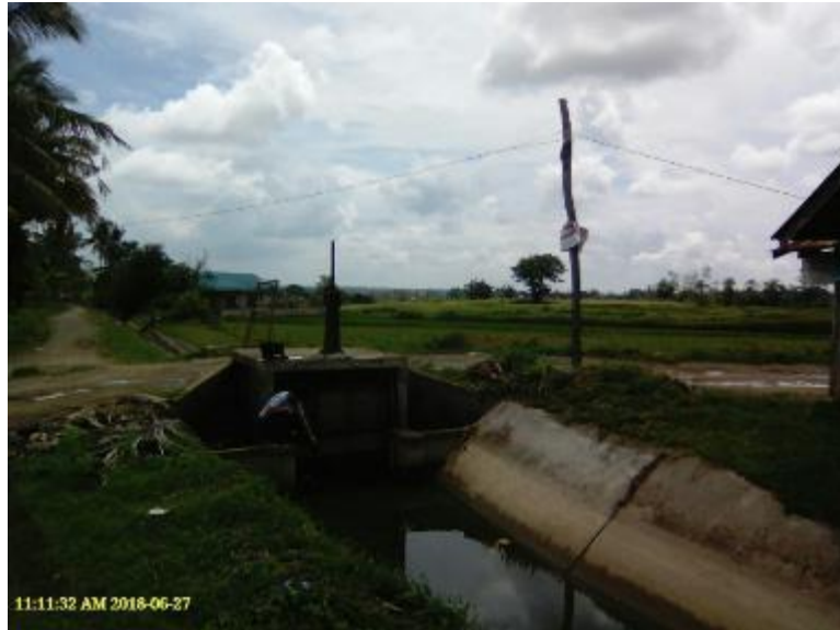
Photo 40. Check gate at the downstream section of Lateral D, Malinao IS. Take note of the debris on both sides of the canal.
