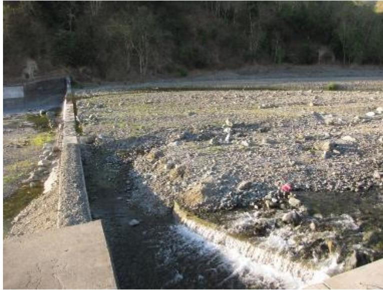
Photo 1. Silted diversion dam of Dipalo RIS
