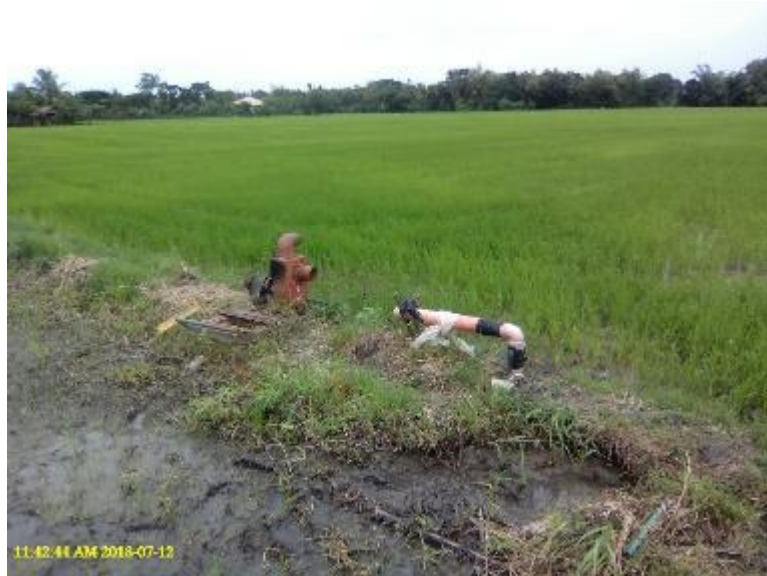
Photo 11. A pumpset installed in the service area of Jalaur RIS (downstream section).
