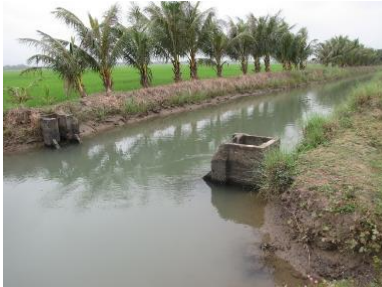
Photo 29. Damaged canal and turnout in a section Lateral Dw-D, Div.4, MARIIS. Take note that the Lateral was unlined
