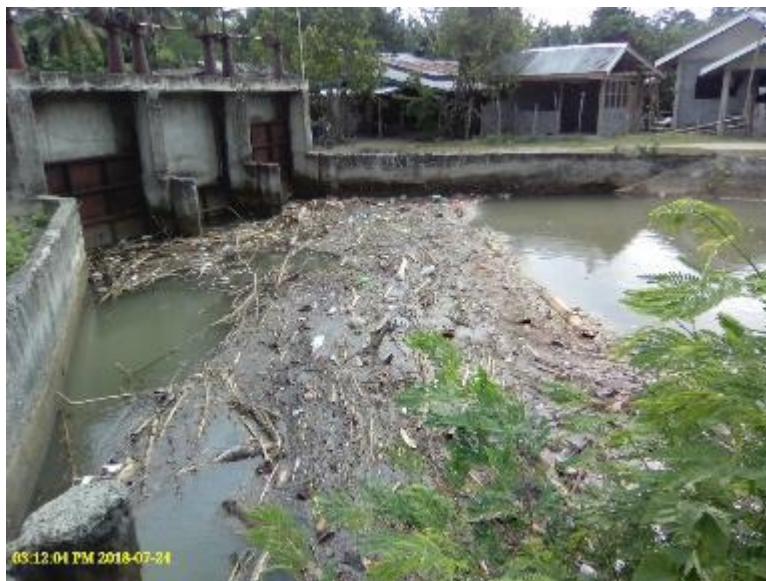
Photo 98. Debris trapped in a checkgate along Main Canal of Malitubog-Maridagao RIS.
