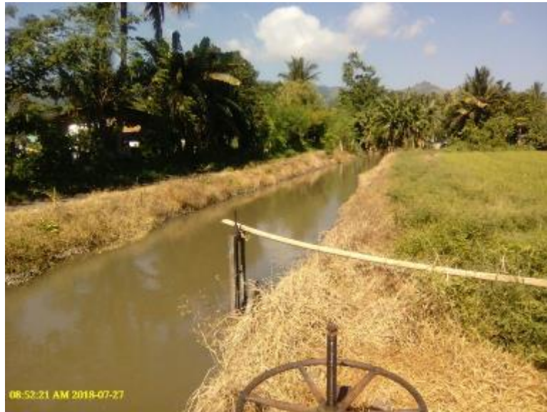
Photo 89. Silted section of Marbel #1 RIS.
