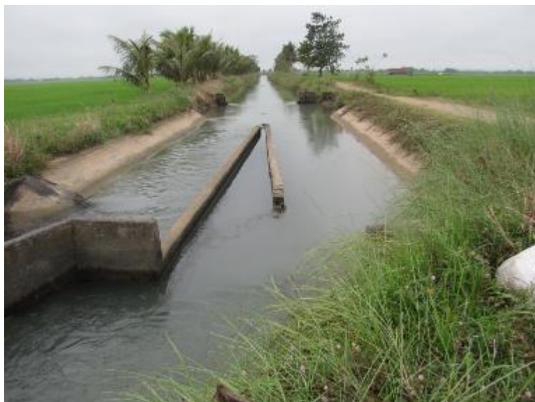
Photo 28. Damaged structures along Lateral D2, Div.4, MARIIS
