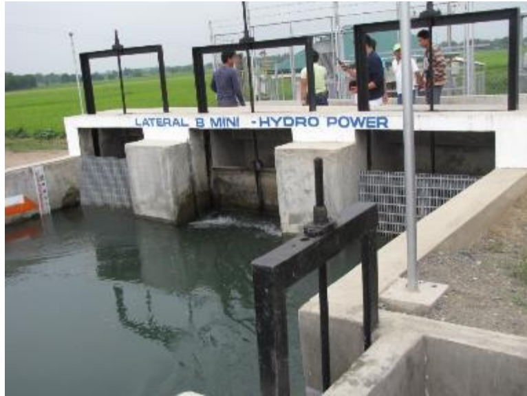
Photo 33. Mini-hydro power plant (45kW) along Lateral B, Div. 2, MARIIS.
