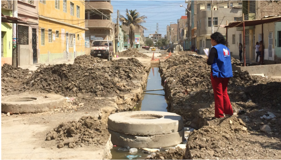
Figure A11: Sewerage project abandoned in Huanuco
