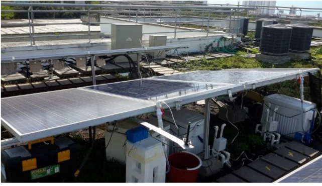
Fig. 3. Irrigation system with two PV panels (P6 and P7) installed on the green roof together with some components of the monitoring system. (For interpretation of the references to colour in this figure legend, the reader is referred to the web version of this article.)
