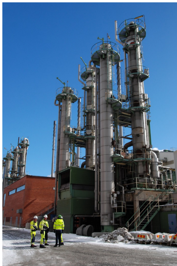
Fig. 1. The four HPC/Benfield CO 2 separation lines at the gas refinery in Stockholm that operated utilizing hot potassium carbonate between 1971 and 2011 (photograph taken 16 March 2018).
