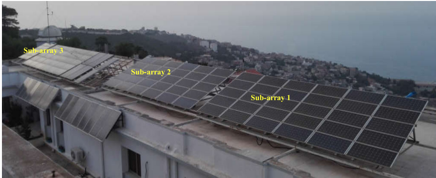
Fig. 4. Grid connected photovoltaic generator on roof.
