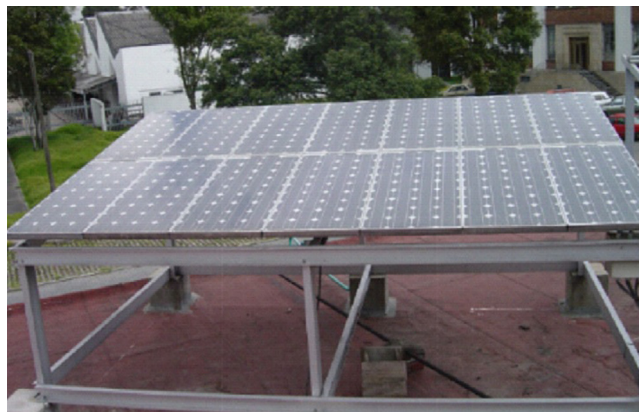
Fig. 2. BIPV system installed in the terrace of the Department of Physics of the National University of Colombia, Bogotá.
