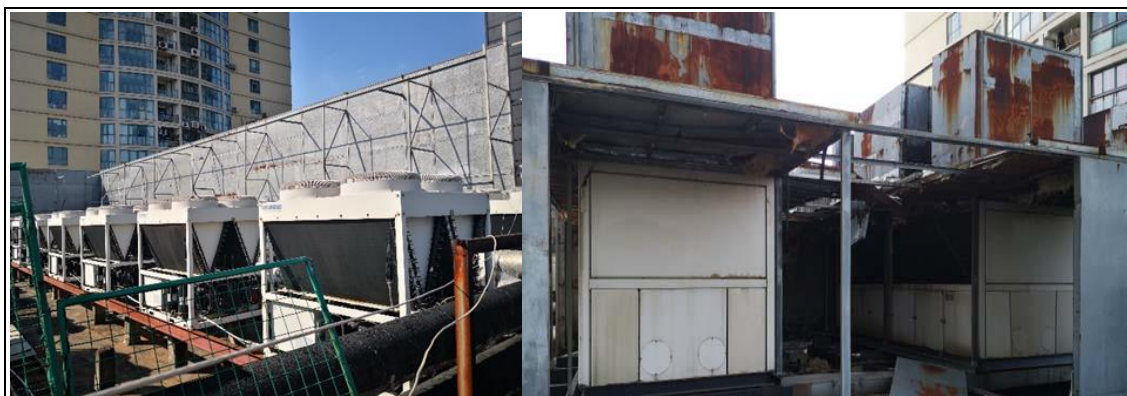
Figure 10: Photo of Air-Conditioning Unit in Ningbo Shopping Plaza
