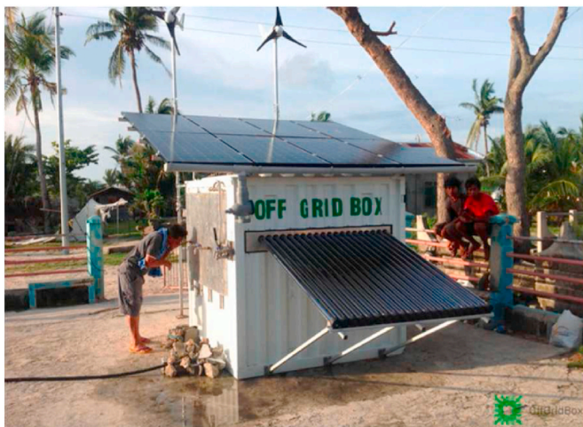
Fig. 1. Off grid box in Gasagara, Rwanda.
