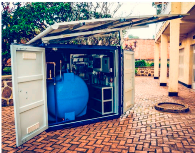
Fig. 5. Pilot design of the water purification system within the OGB system. It is composed of a 5- \mu m filter and an activated carbon/charcoal filter and an ultraviolet (UV) lamp. It also has a desalination option. The input sources can be rainwater, municipal water, groundwater, or freshwater. The clean water can then be distributed in jerrycans, sachets, a smart-tap, or packaged water.
