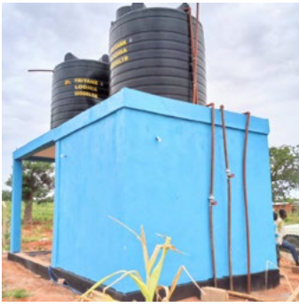
Left: Raised water tanks at Kisisi borehole, Mpwapwa, Tanzania, 2023. Photo: Peter Msumali Rogers
