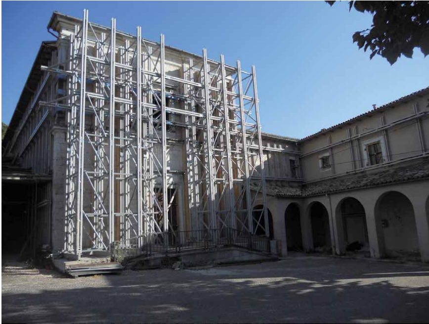
Figure 11. Shoring of the church of the Convent of Santa Chiara (photo S. Gizzi, 2011).
