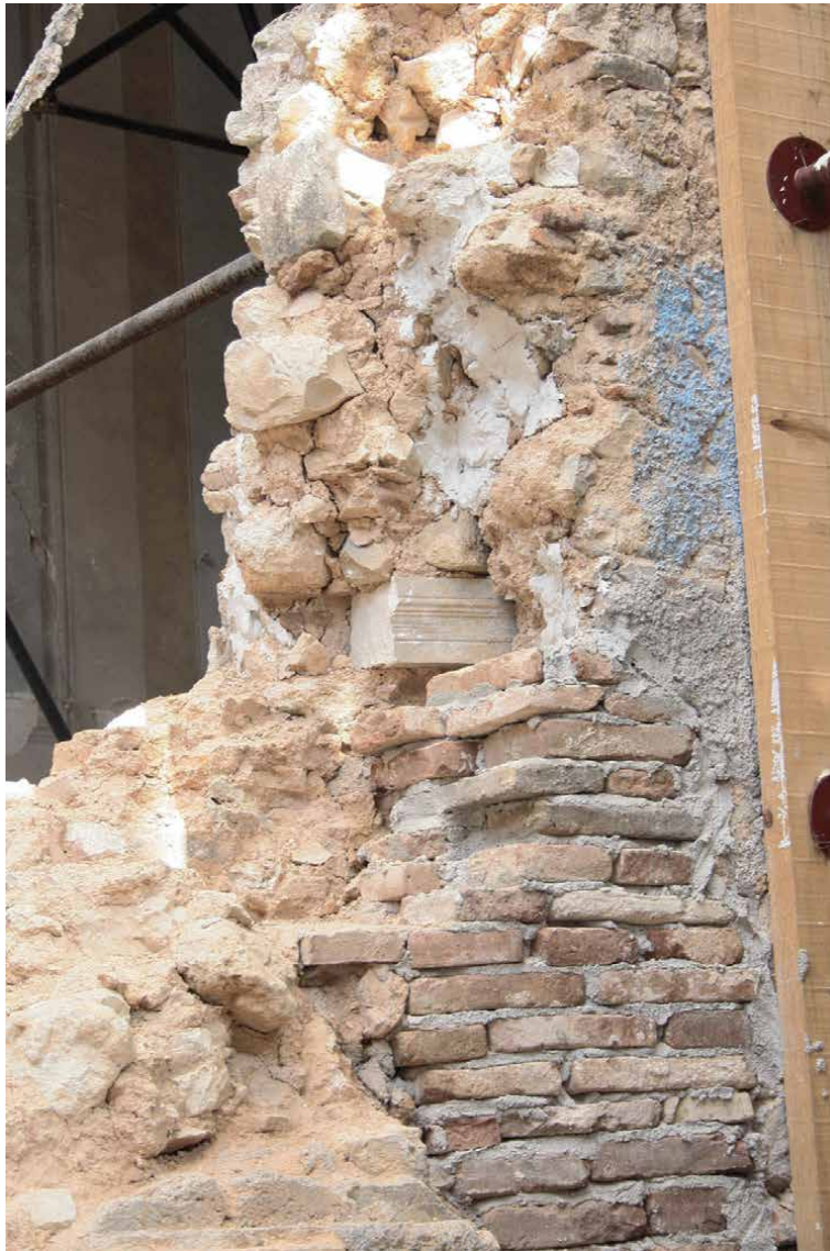
Figure 37. L'Aquila, church of Santa Maria Paganica. Reused stone elements that came to light inside the eighteenth-century walls after the collapse (photo S. Gizzi, 2010).
