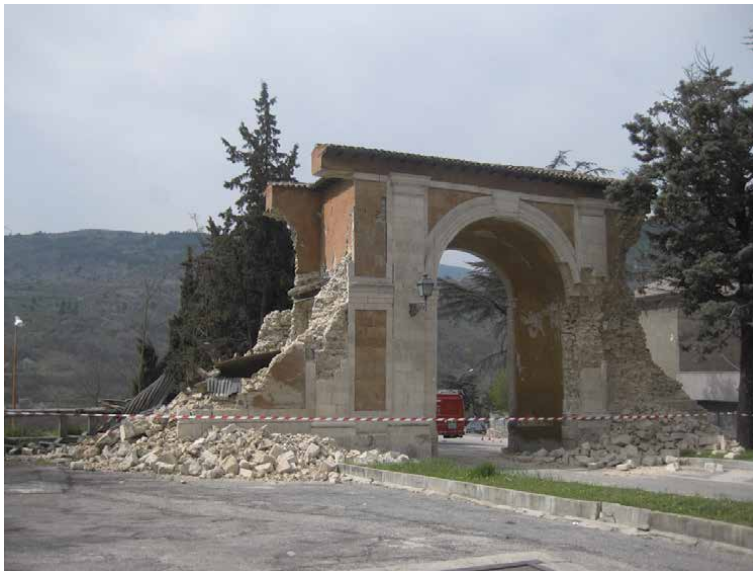
Figure 30. Porta Napoli, at the end of Corso Federico II, immediately after the partial collapse (photo S. Gizzi, 2009).
