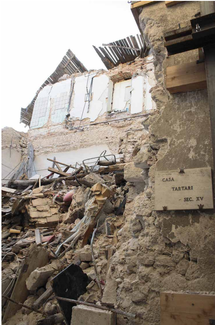
Figure 32. L'Aquila, collapses in the historic center: Tartari house, from the 15th century (photo S. Gizzi, 2010).
