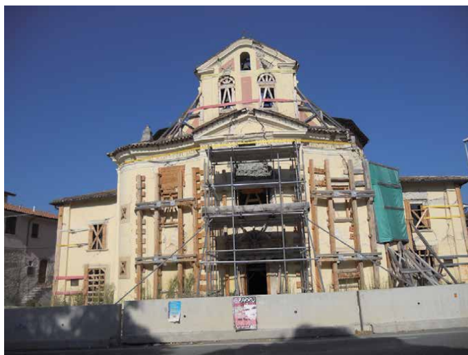
Figure 14. Emergency provisional works in wood in the church of Paganica (photo S. Gizzi, 2011).
