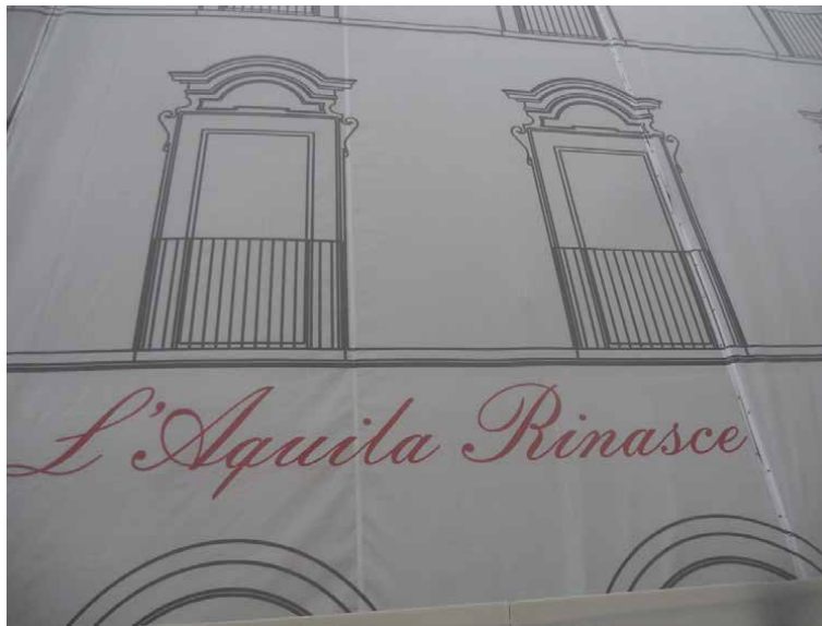
Figure 38. The words “L'Aquila is reborn” on a restoration site scaffolding (photo S. Gizzi, 2014).
