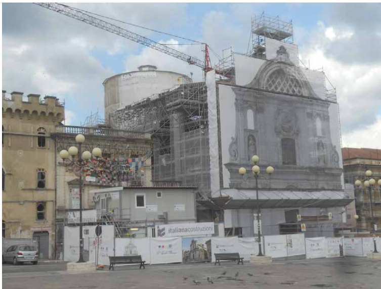
Figure 19. The church of the Holy Souls (Santa Maria del Suffragio) in Piazza Duomo in L'Aquila in August 2014 (photo S. Gizzi, 2014).
