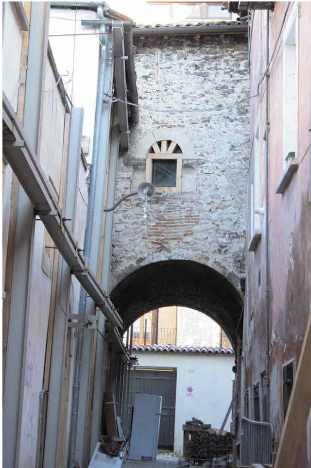
Figure 13. “Provisional works in one of the alleys in the quarter of San Pietro di Coppito in L'Aquila” (photo S. Gizzi, 2011).
