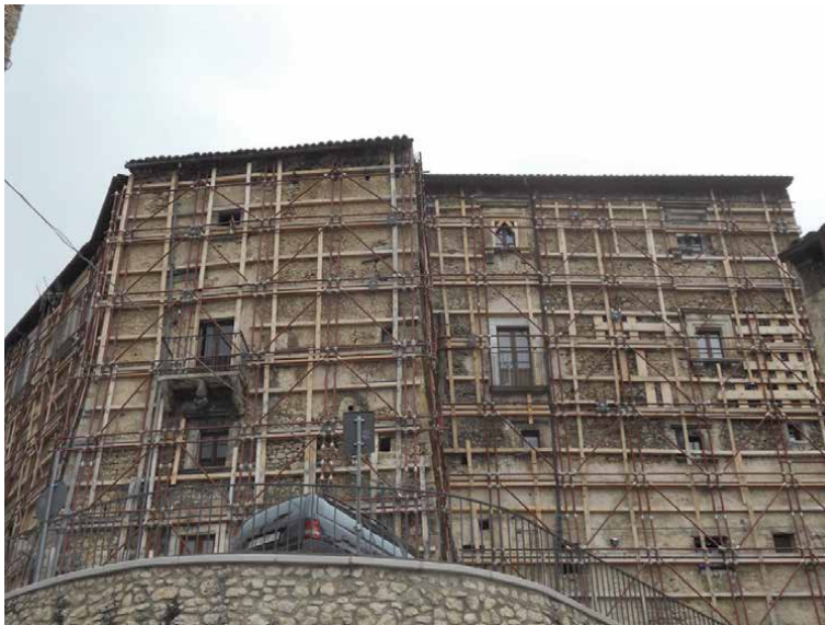
Figure 16. Provisional wooden work and props in the Medici center of Santo Stefano di Sessanio, near L'Aquila (Photo S. Gizzi, 2011).
