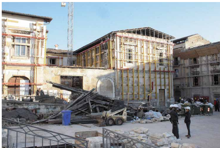
Figure 18. Props, temporary coverings and temporary works of various kinds in the square of San Pietro di Coppito in L'Aquila (photo S. Gizzi, 2010).
