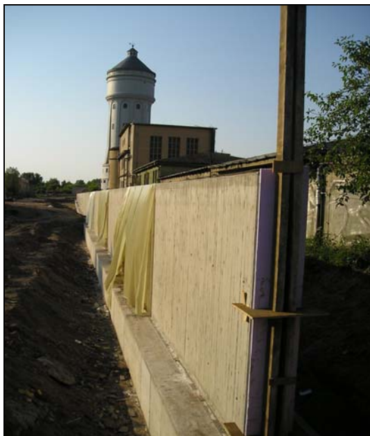
Photo 1: Flood Wall in Front of the Former ECW; Source: Kuhlicke 2008
